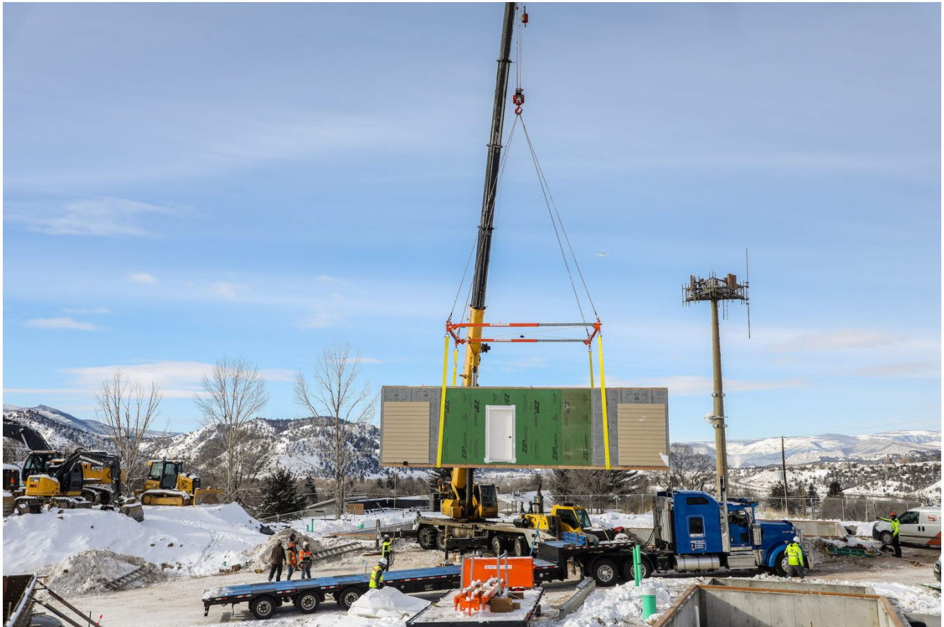
A crane lifts a section of a modular home being installed at the Habitat for Humanity Third Street project Tuesday in Eagle.
