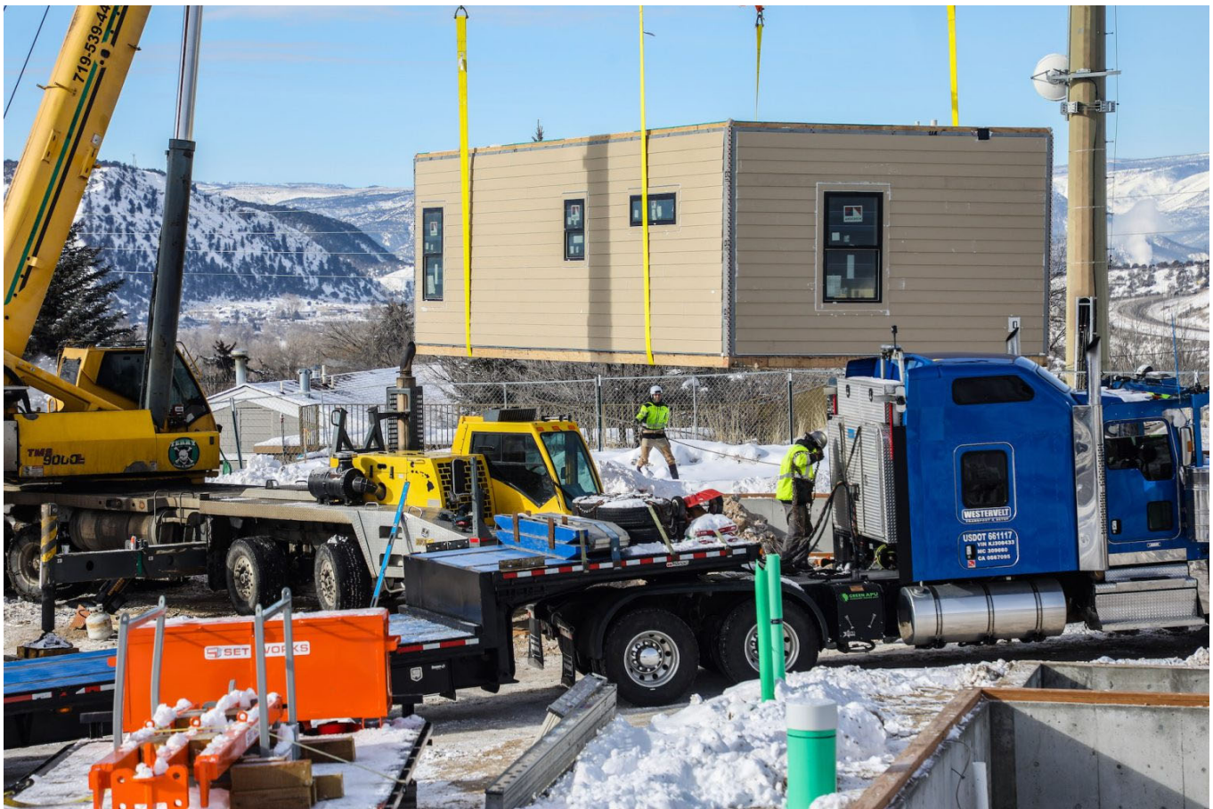
Part of a modular home is set on a foundation during Tuesday's craning-in event for the Habitat for Humanity Third Street home project in Eagle. ThirdStreet-VDN-011824-6
